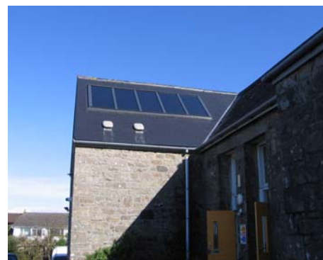
Left: Sunslate Solar PV tiles installed by Plug into the Sun at Carnyorth Outdoor education Centre.
