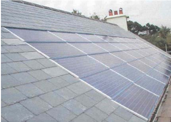
Solar PV at the Centre of Pendeen
